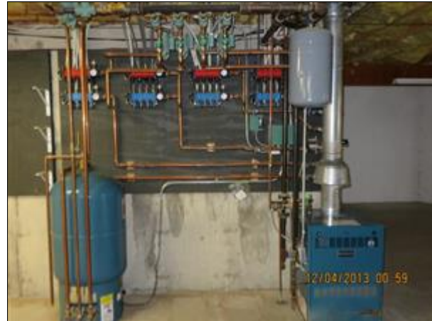
Radiant heating system
