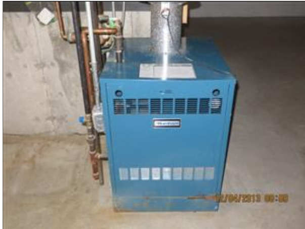
Propane gas FHW boiler
